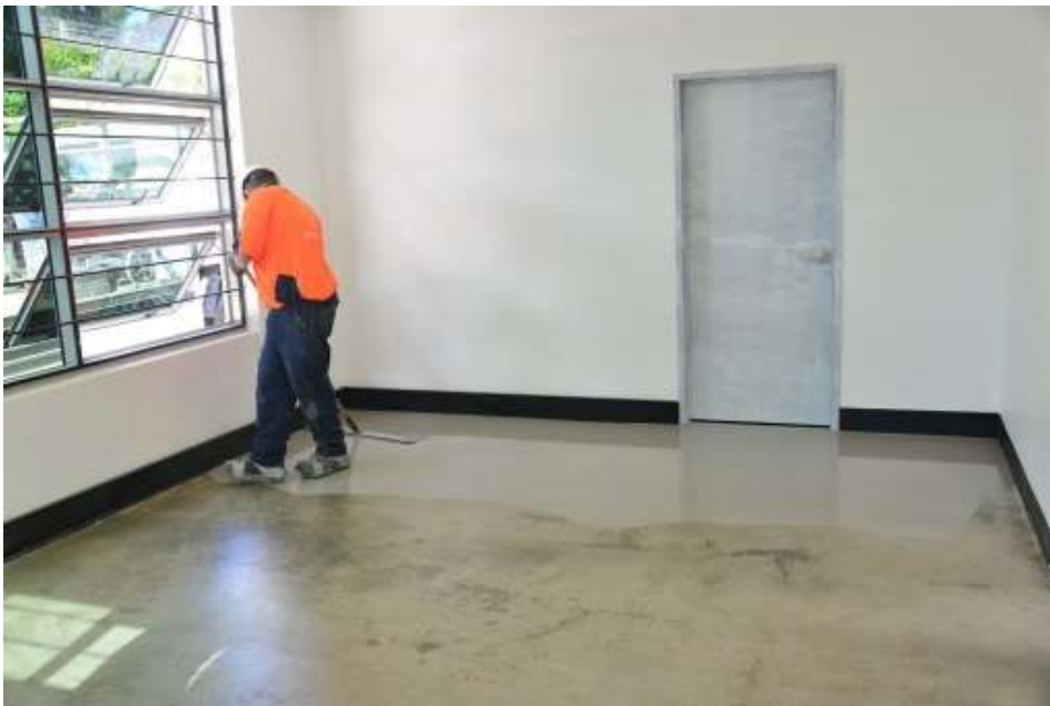
Figure 5 After pouring from Hippos spread over the floor to ensure it gets to all corners
