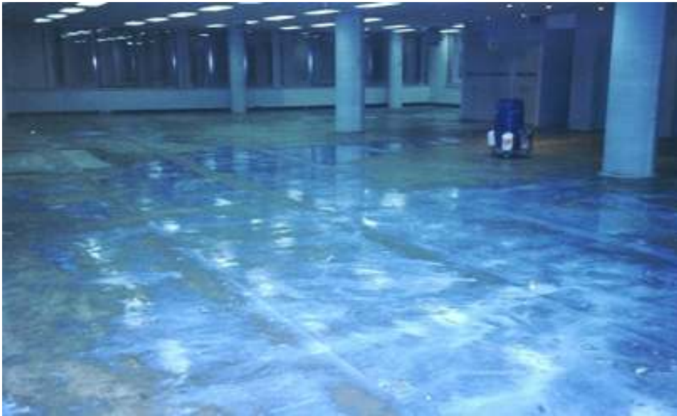
Figure 2 Once prepared and vacuumed the primer can be applied to seal the surface
