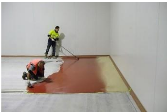
The concrete slab floor was first shot-blasted and had minor repairs made, prior to a 9mm thick trowel application of Ucrete DP20
