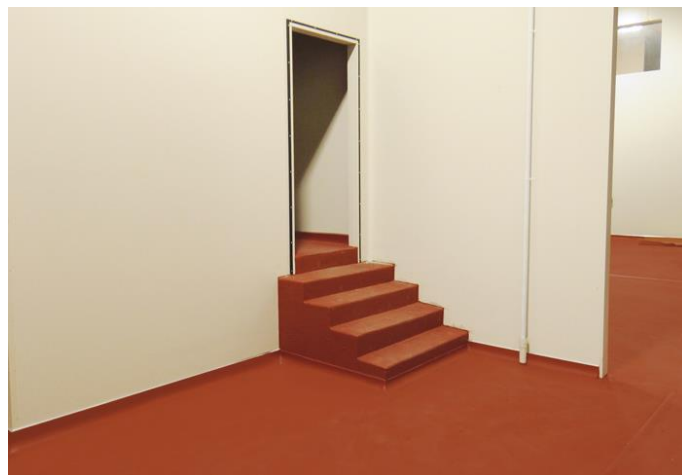
Approximately 1,000m 2 of Ucrete DP20 was used in PMF's Homebush Bay prepacked fresh soup and salad processing and packaging facility
