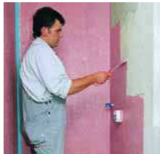
2. Apply undiluted MasterTile WP 668 (red) to the substrate as a first protective coating to cover its entire surface.
