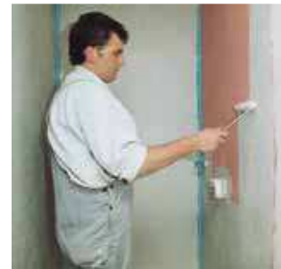
5. After an evaporation time of approx. 1 hour apply the second protective coating with MasterTile WP 668 (grey). The first coat of MasterTile WP 668 (red) should not be visible, otherwise another layer might be necessary.
