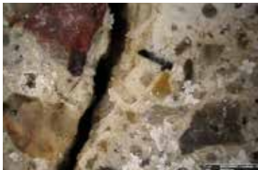
Magnified hairline crack in concrete
